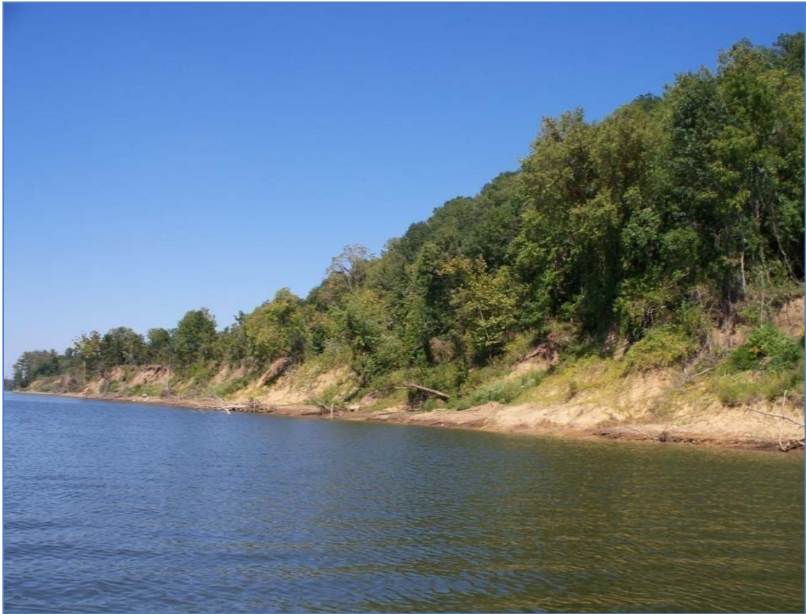
Figure 4-16 Cumberland River Embankment Needing Riprap
